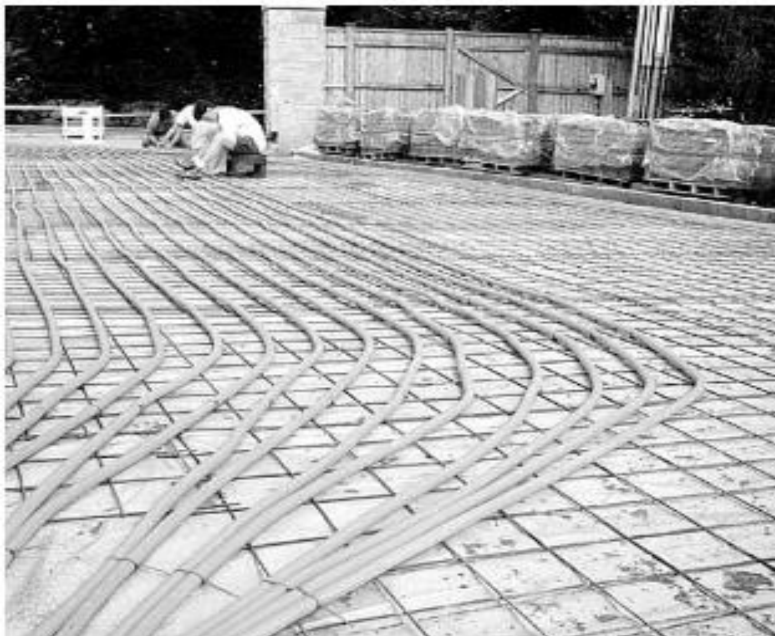
Figure 4. The heating system is tied to a wire mesh anchored into the compacted aggregate base.
